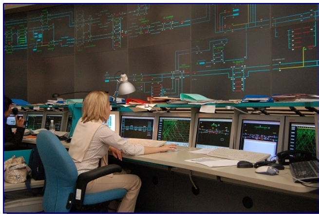
Figure 1. Operator and synoptic frame in Genoa’s SCC.
